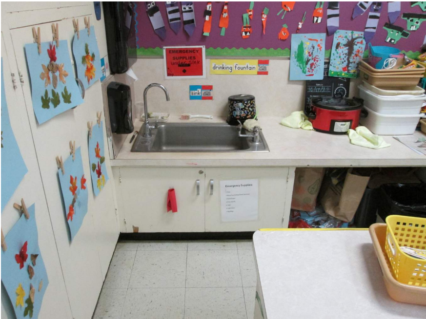
Accessibility upgrades required
