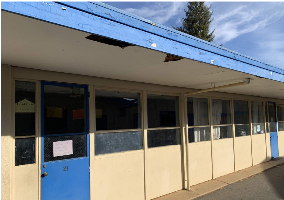
Exterior finishes need repair or replacement
