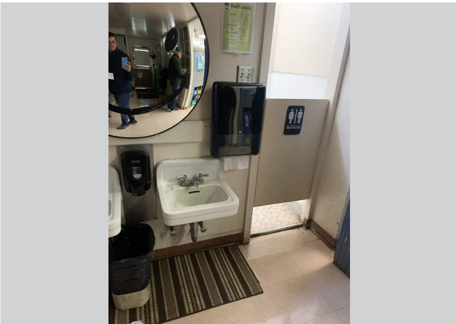
Restroom upgrades needed for ADA compliance
