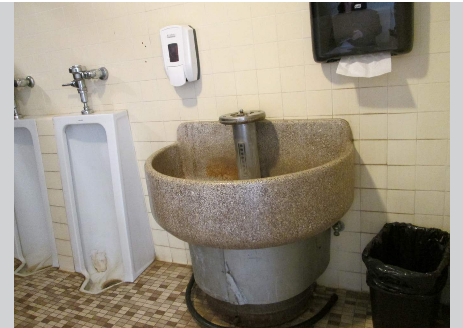
Restroom plumbing fixture replacement needs and ADA compliance
