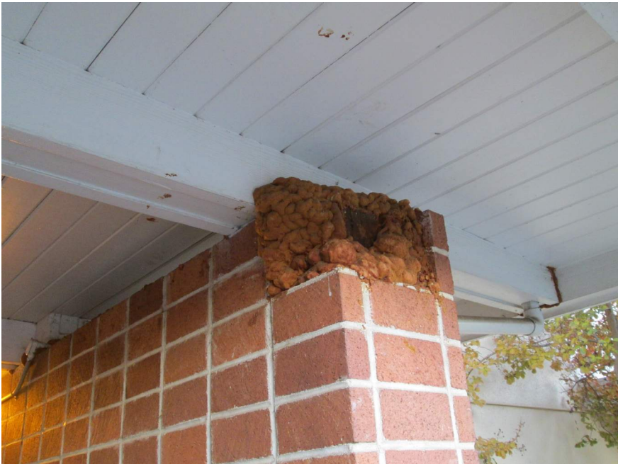
Ongoing deferred maintenance
