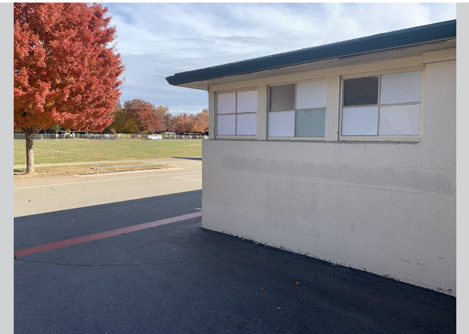
Exterior paint and window replacement needed
