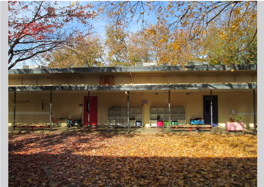
ADA path of travel upgrades to pavement and thin metal doors
