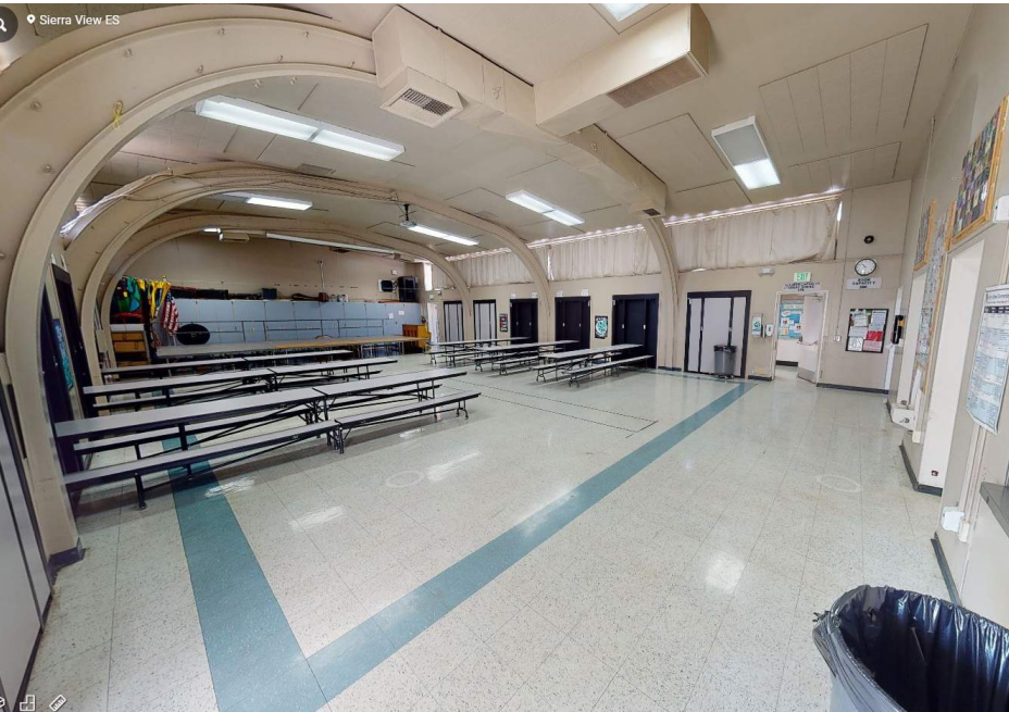
Multi-purpose room upgrades needed
